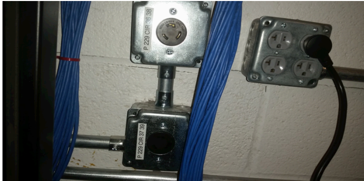
Two 220 Volt Connections
